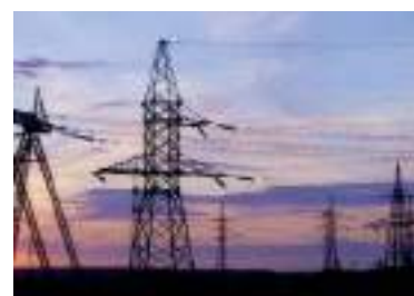
High Voltage Lines Management System
